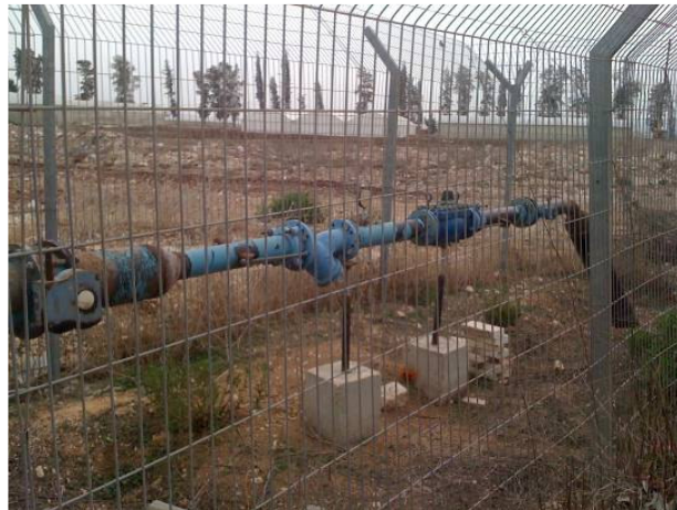
Mekorot line in Jalama.
